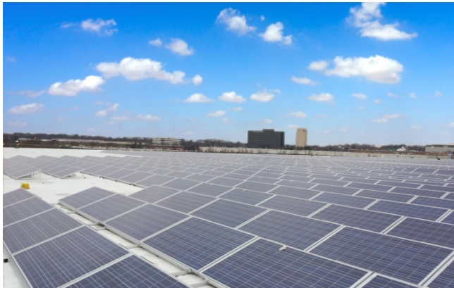
Macy's, New Jersey, USA 1.1 MW Project
